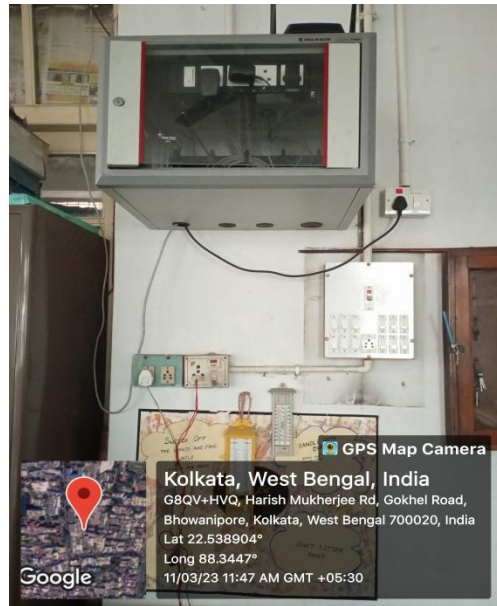
Wi-Fi Control Panel
